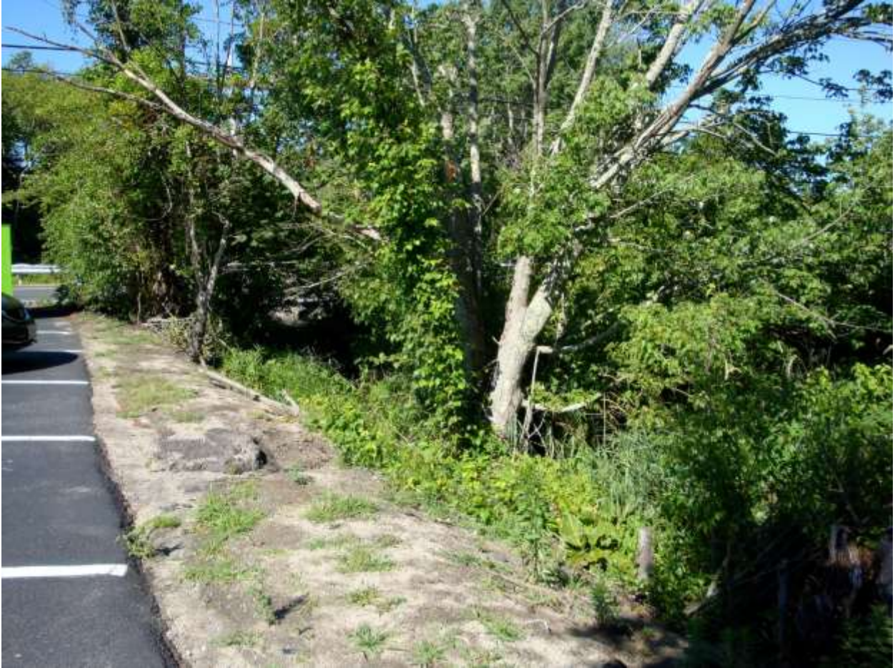
4444 parking lot with eroded bank (approximately 12 spots in length to the right of green bin)
