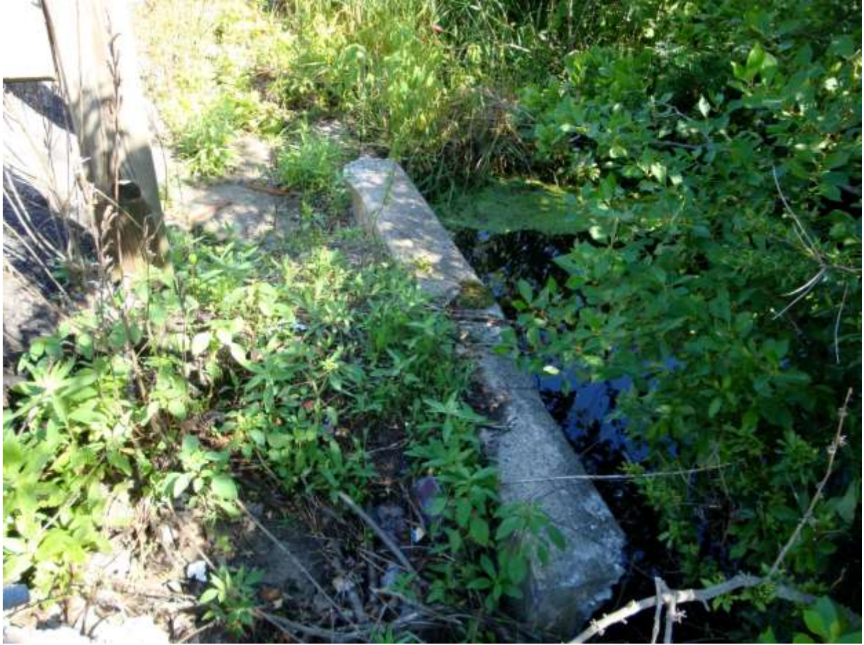
4449 monitoring site - side view of concrete outfall - brook runs behind Morris Farm under Rt. 117A to monitoring site
